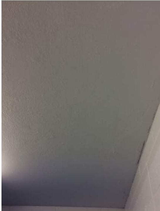
Photo 29: View of Homogenous Area 29 FMS Room 109
